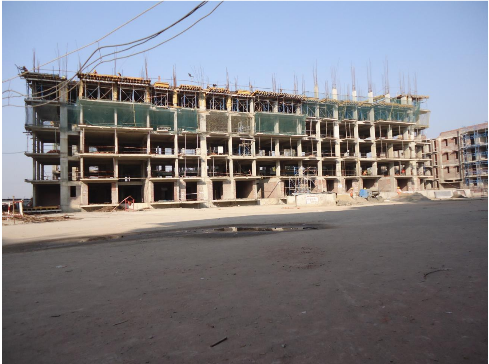
Juniper Court - Fourth & Fifth floor roof level slab & column work in progress Mid Rise N (Block 6)
