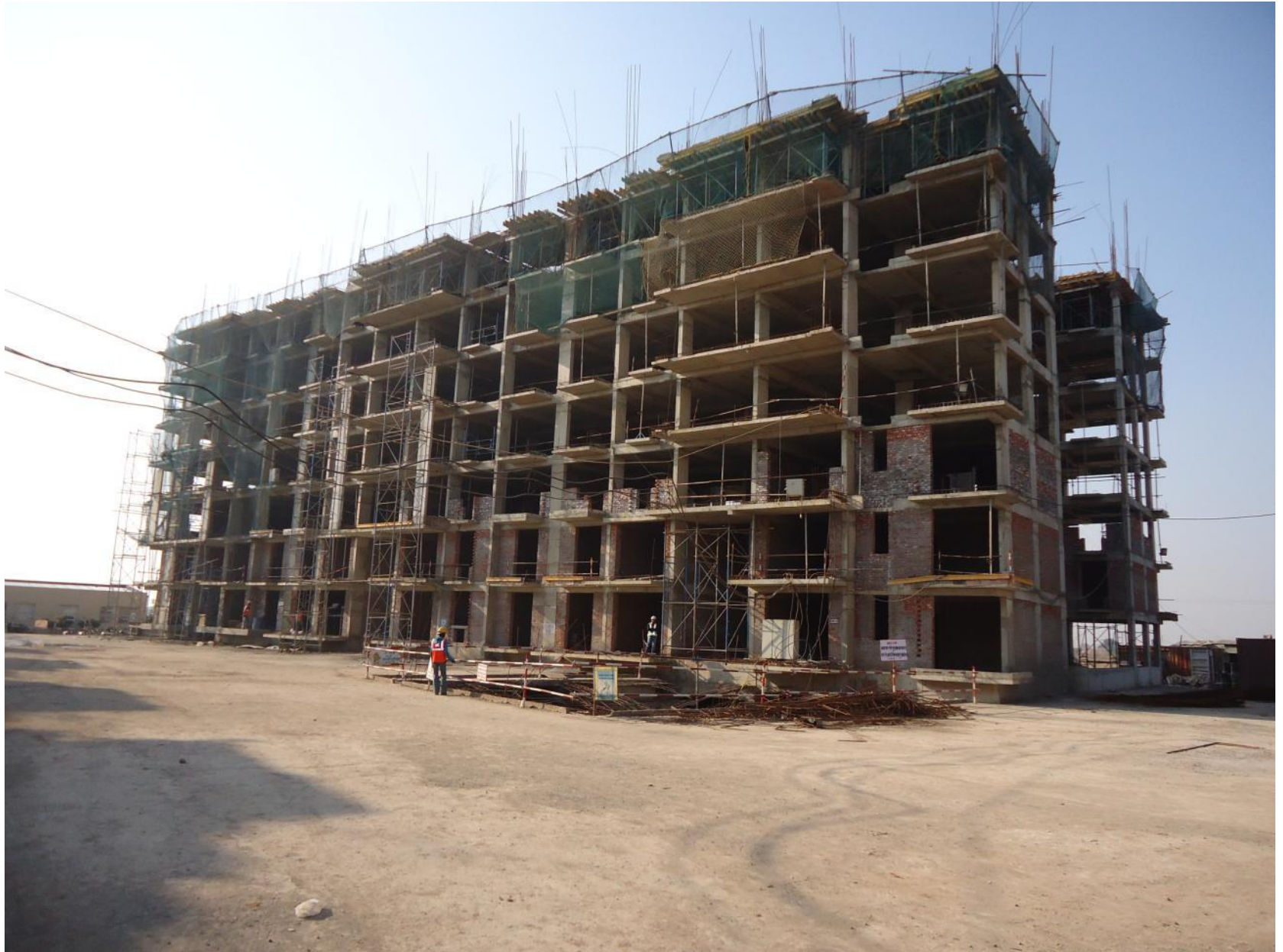
Frangipani Court - Sixth floor level roof slab completed & brick work in progress Mid Rise W (Block 5)
